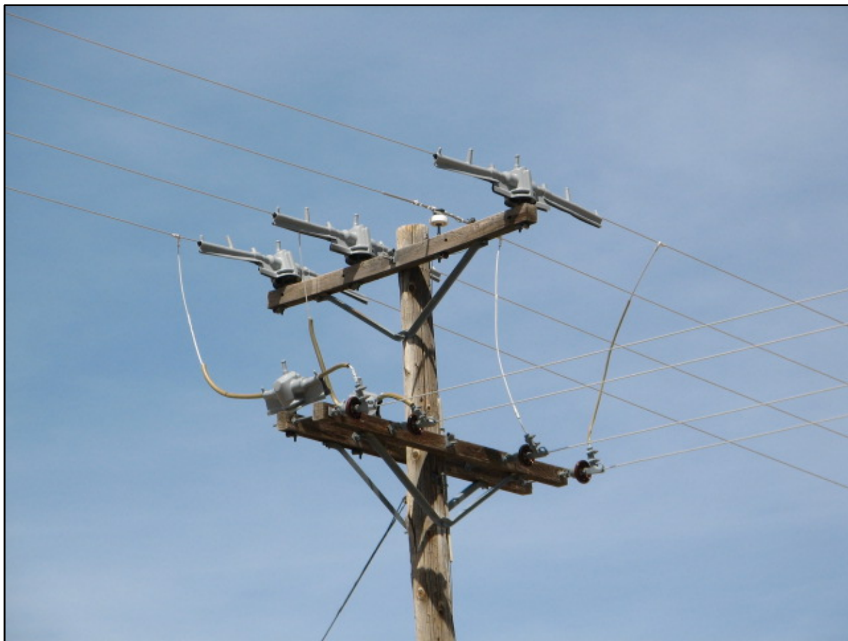
Figure 6-3. Retrofitted pole with conductor wire covers, insulator covers, and extenders.
