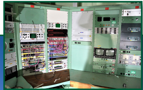
Control panel on 3rd floor of EMAD
