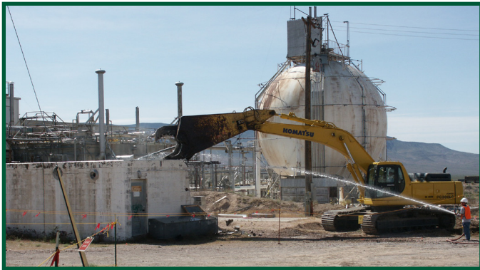
A worker sprays water for dust suppression as a worker using hydraulic shears dismantles a building at the Test Cell A Facility on the NNSS
