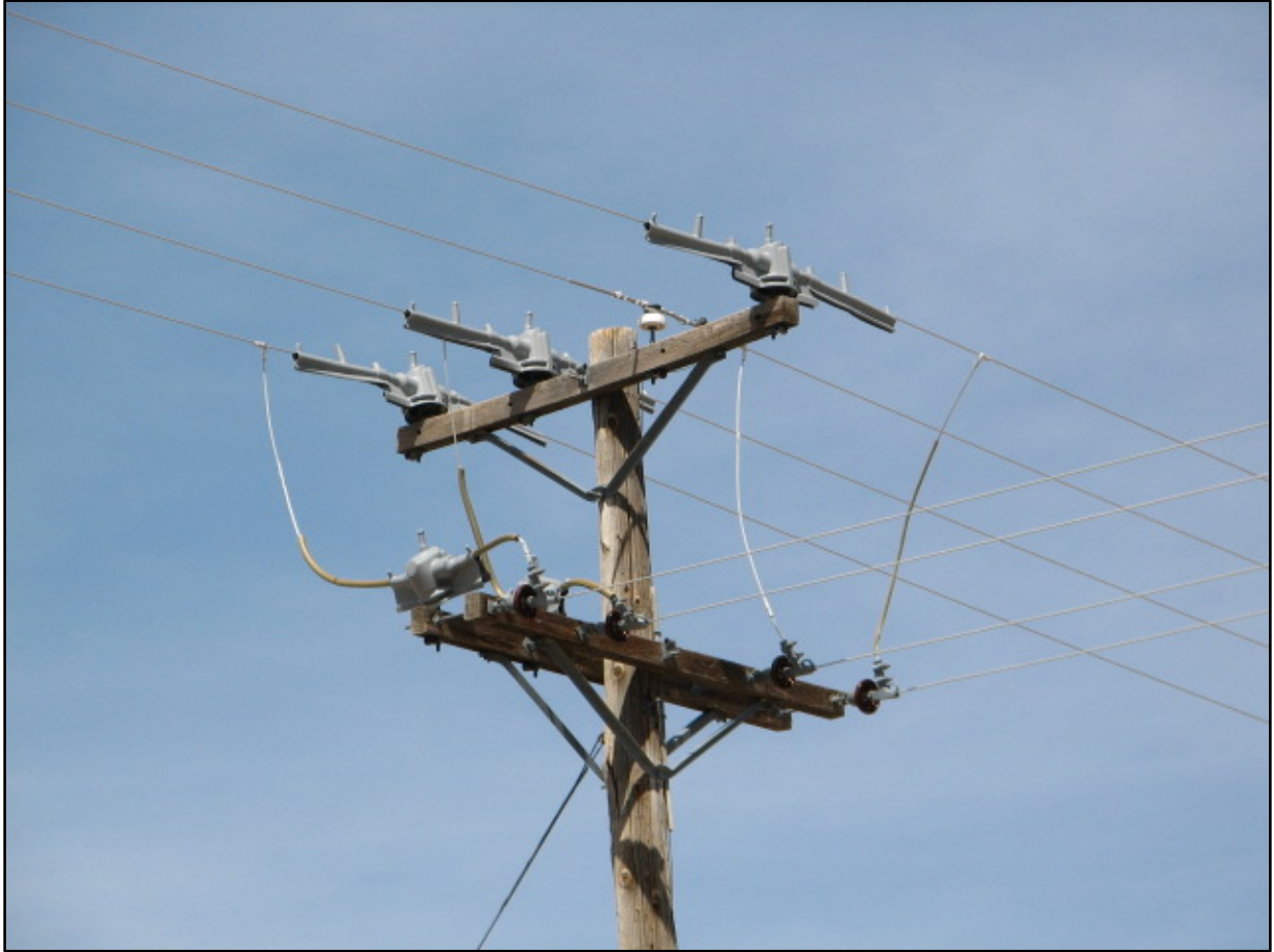
Figure 6-2. Retrofitted pole with conductor wire covers, insulator covers, and extenders.
