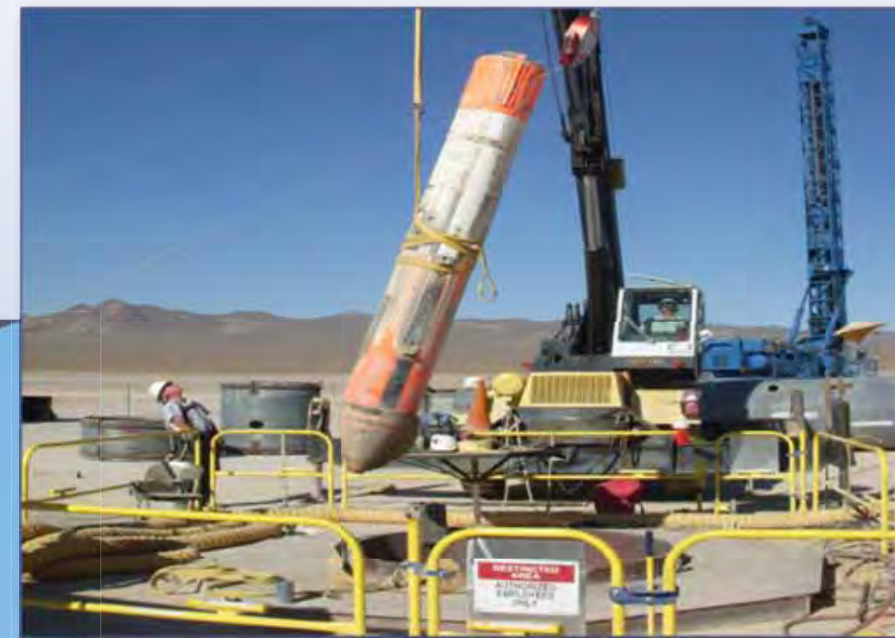
Post-test activities include excavation and recovery of the buried B83 Joint Test Assembly
