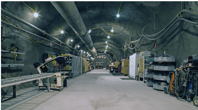
Underground tunnel at the U1a Complex at the Nevada National Security Site.
