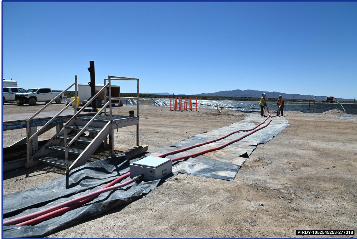
Rolling Out Bypass and Discharge Lines (Including Flowmeter) to Sump at ER-20-1 (May 4-8)
