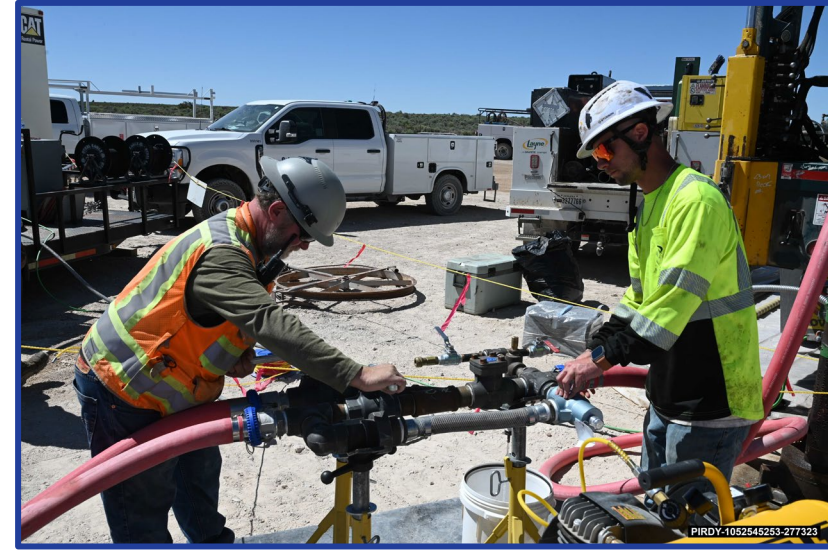
Adjusting Sampling Manifold Valves at ER-20-1 (May 4-8)
