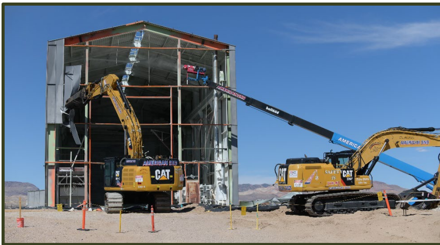
Left: Crews began work to remove the siding on the south side of the trainshed at EMAD Facility at the end of March 2025.
