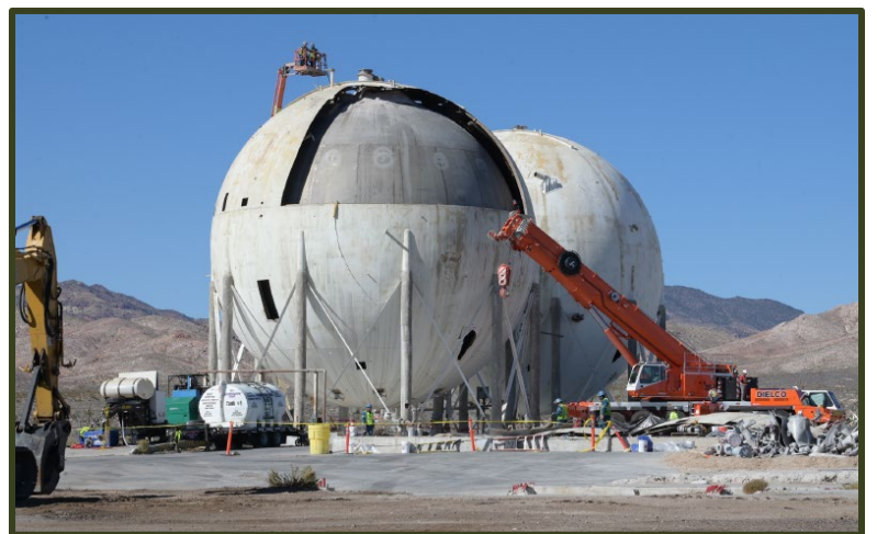
Right: Size reduction work is underway at larger Dewars 1 and 2 at the TCC Facility.
